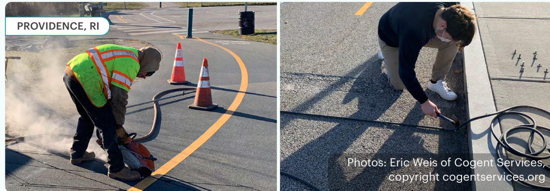
Saw-cutting pavement to install in-ground inductive loops to count bikes on Gano Path. Installing pneumatic road tubes to count bikes on a 2-way cycle track on Clifford St.
